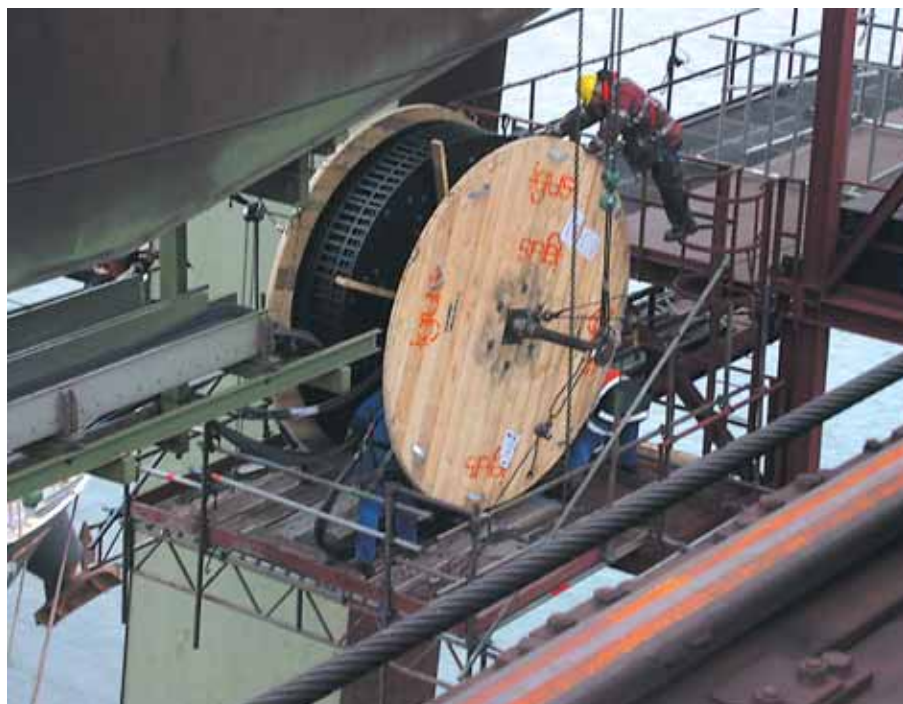
ReadyChain® installation by igus® supervisor on a bulkhandling Crane. Weight of the E-Chain® incl. Chainflex® more than 2 t.
